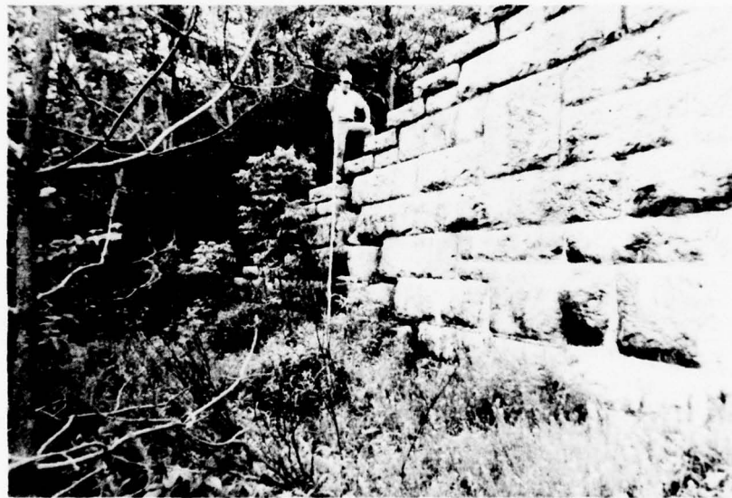
D. Crack at Downstream Toe of Retaining Wall
